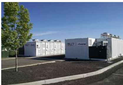
Energieopslagproject in Pullman, VS (Foto: UniEnergy Technologies)
